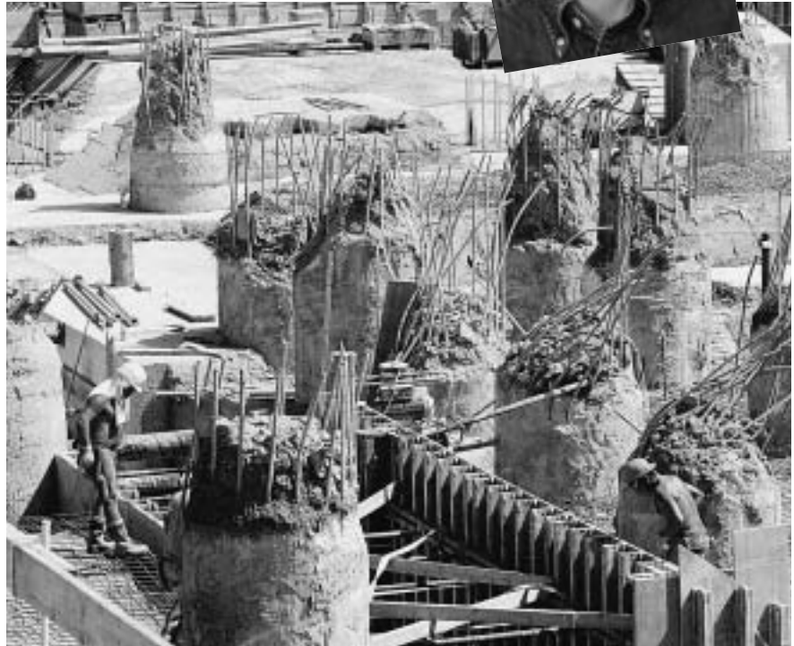
The Zurich "energy piles"
